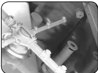
Stainless steel wash tank
